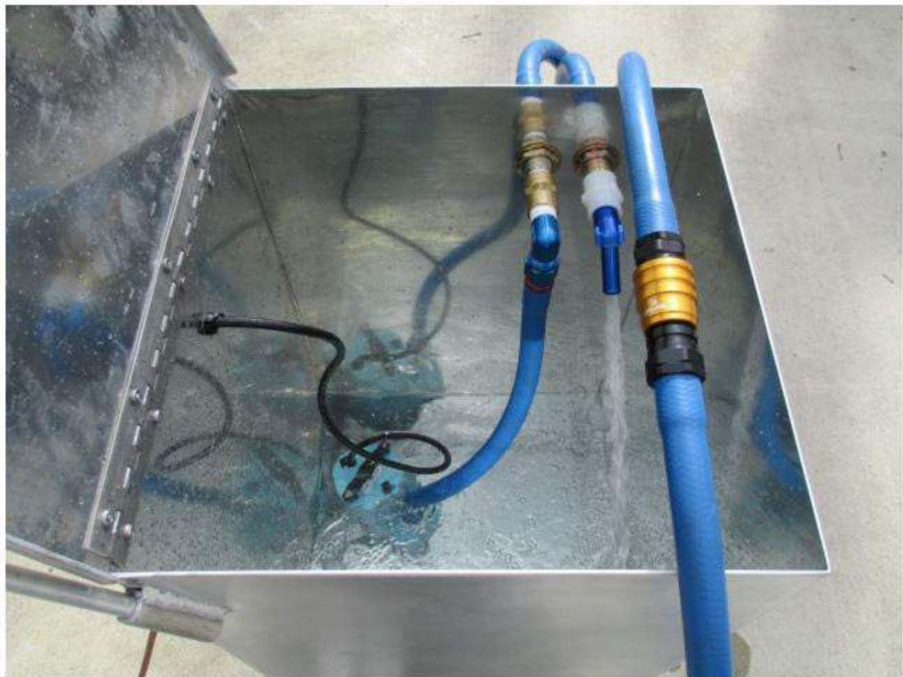
The chiller in operation – the ice water mixture is pumped out through the left hose and returns to the tank through the inlet on the right.
